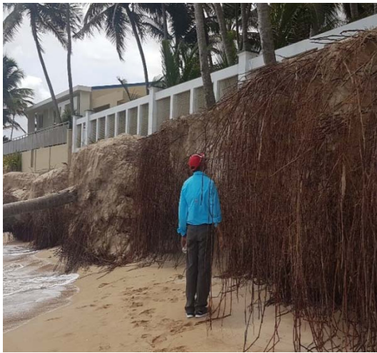
Figure 4. Vertical cut produced by wave impact during the second week of August 2019. Source: Méndez-Tejeda
